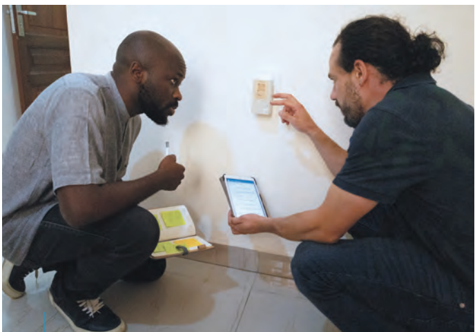
Samuel Miles and Emery Mbavumoja of the Congolese Rural and Peri-urban Electrification Agency install a sensor that monitors power quality and reliability.
